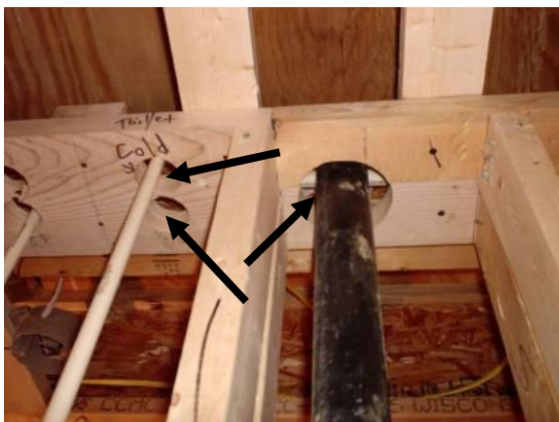
-seal all penetrations through the top sill plate on walls. (missing in photo)
