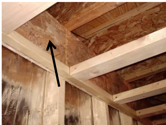
-plywood used as fireblocking from the soffit to the wall cavities.
