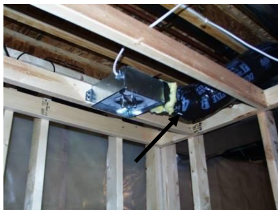
-insulated flex duct from bath fan leading to exterior, minimum 3 feet from exterior wall in required to be insulated.
